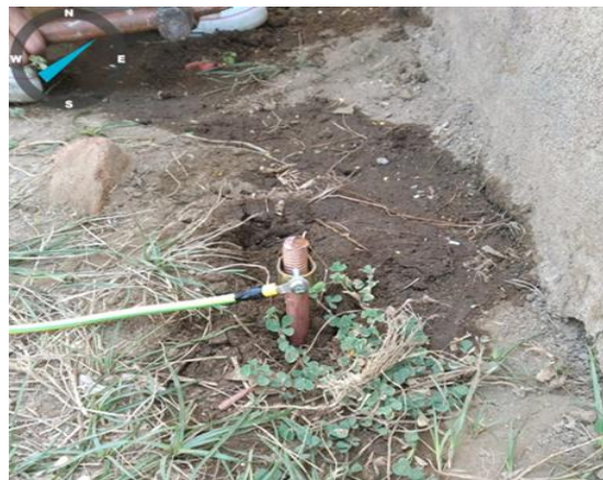
Figure 3.3. Grounding and grounding cable
