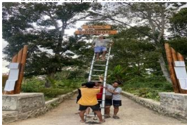
Figure 2. Repairs to the Gate at the Entrance Area of the Sumberan Camping Ground
